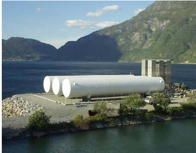
Figure 8. Large satellite plant, 1500 m 3 storage, 4400 Sm 3 /hour vaporization
