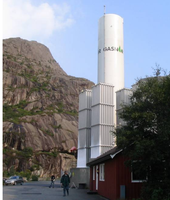
Figure 7. Medium Satellite plant 257 m 3 storage, 1500 Sm 3 /hour
