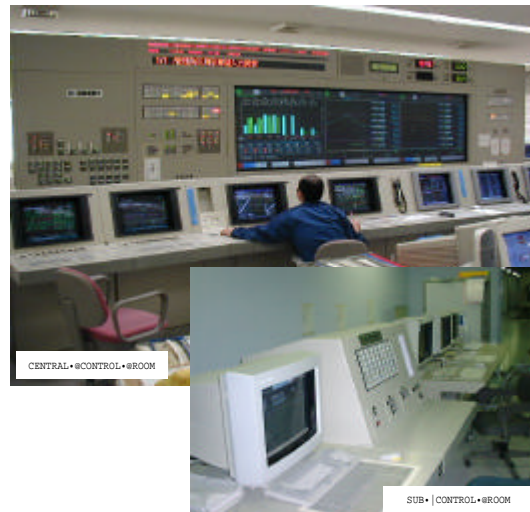
Fig.10 Central Control Room and Sub-control Room
